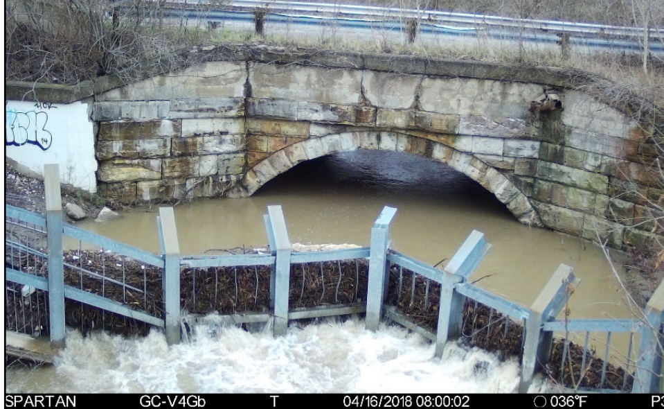
April 16, 2018: Peak Storm and Debris Accumulated on Rack
